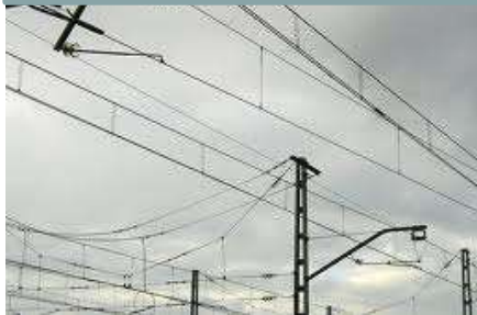
OVERHEAD CONTACT LINE
