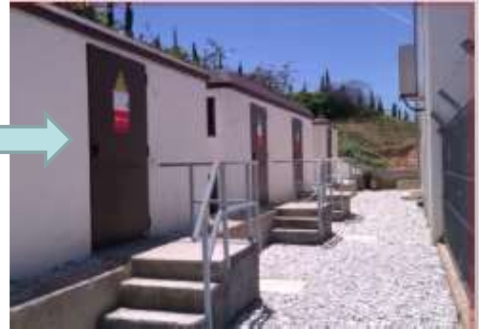
INVERTER IGBT, 1 MW
